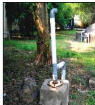
Fig. 3.1.4. Auto distribution system for roof water runoff
