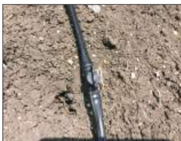
Individual control system
