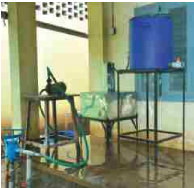
Organic fertigation unit
