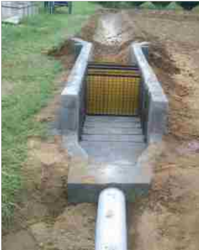
Plate 3.1.2a. Composite filter installed in field laboratory
