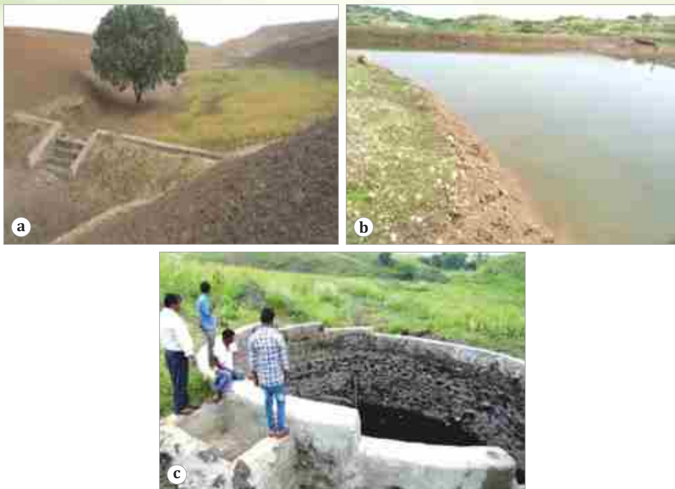
Plate 4. Low cost water harvesting structure (a & b) and monitoring of water table in a well near the structure (c) at village-Doongri pada, district-Banswara, Rajasthan
