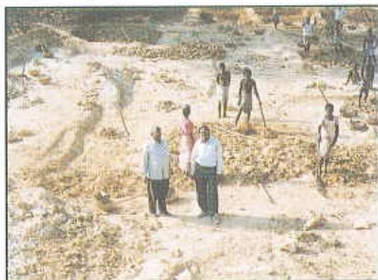
Photo 2 : Construction of tank in progress (No machines were used for earthwork to increase the employment generation)
