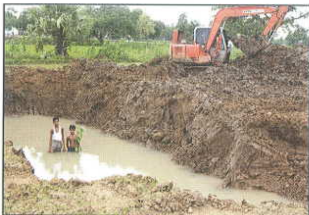
Photo - 5 (a) : Digging of pond in progress in land with shallow water table
