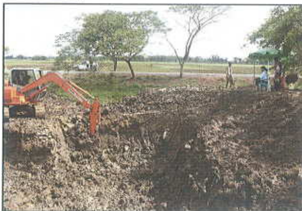
Photo - 5 (b) : Digging of pond in progress in land with deepwater table
